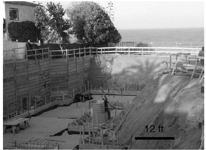
Excavation for a house under construction on Ocean Avenue. The depth of the excavation is approximately 20 feet. Note pilings and shoring near neighboring property at the left (south) of picture. Picture courtesy of Art Olson.
