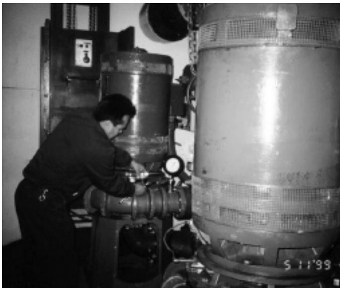
Inside the 21st St. pump station.
